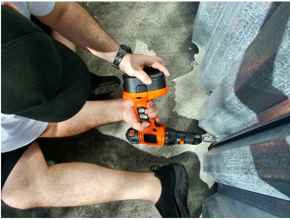
When preparing for an oncoming storm (shown above), be sure there is sufficient staff and time available to install shutters, plywood, or panels.
