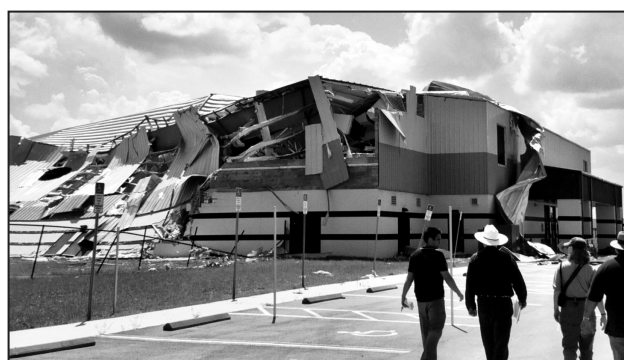
Figure 1-3. Severely damaged hurricane shelter at Turner Agri-Civic Center, Arcadia, Florida (2004)
