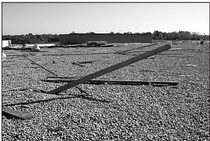
Figure 7-1. Examples of large debris generated by tornadoes and hurricanes
