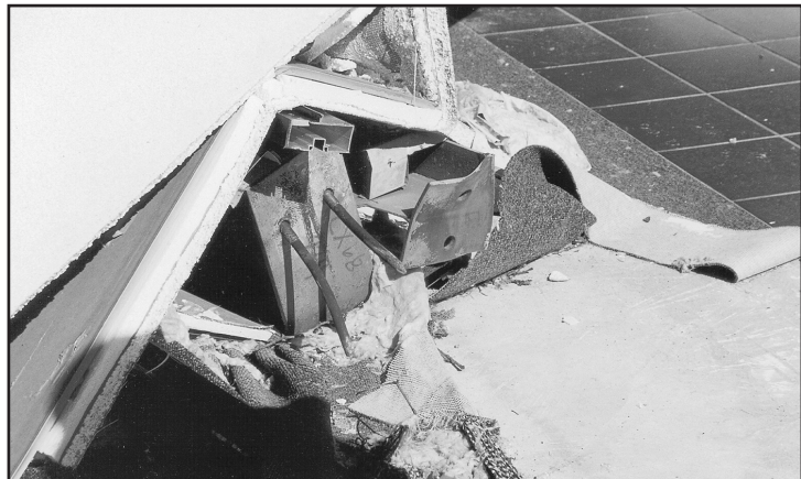
Figure 6-6. These two steel columns failed at their connection to the foundation. The anchor bolts that secured the column released from the concrete (embedment failure) while the anchor bolts that secured the column on the right experienced a ductile failure.
