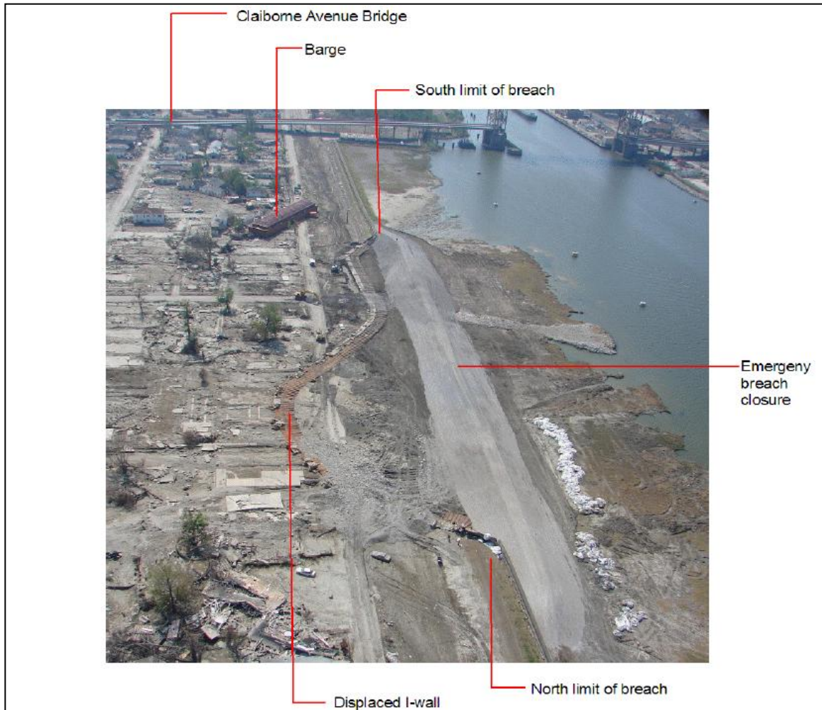
Figure 6-32 Industrial Canal; South Breach at the Lower Ninth Ward; emergency closure (Source: National Science Foundation - Preliminary Report on the Performance of New Orleans Levee System in Hurricane Katrina)
